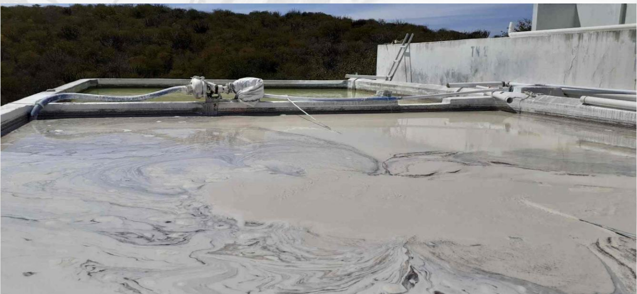
Figure 11 - Flocculation and sedimentation
