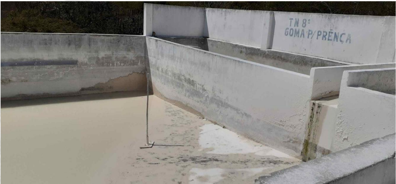
Figure 12 - Gum tanks for presses
